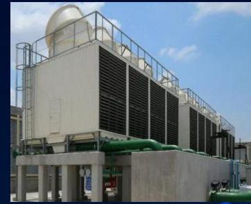
Cooling Towers: 18 nos.
