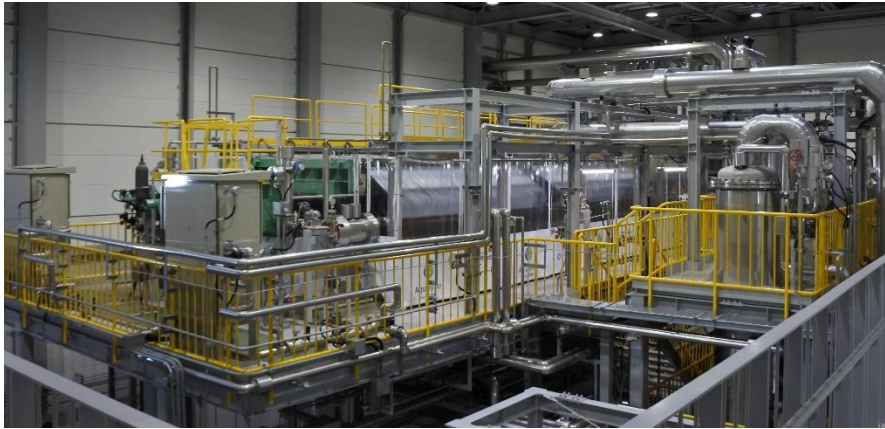
Figure 17 Hydrogen electrolysis of 10MW Fukushima plant 72
