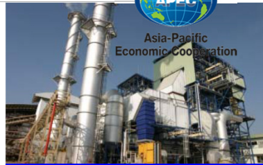
Bagasse Fired Cogeneration (on-grid 29MW) - Phu Khieo Bio-Energy Co. Ltd. Thailand Photo courtesy by COGEN 3 Info Sheet
